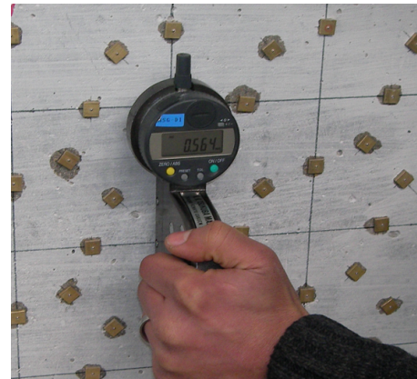
Fig. 4 Monitoring of shear crack displacements by using demec points strain gauge.
